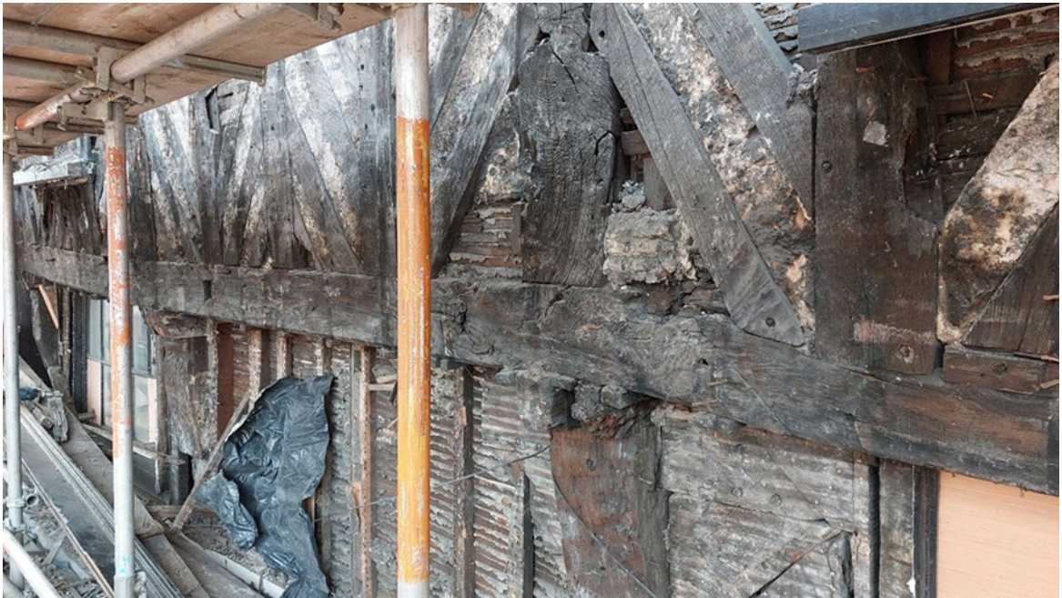
Figure 3: South wall at first-floor level, showing the timber framing of bays 3 and 4, photograph taken from the south-east. [Photograph: Robert Howard]
