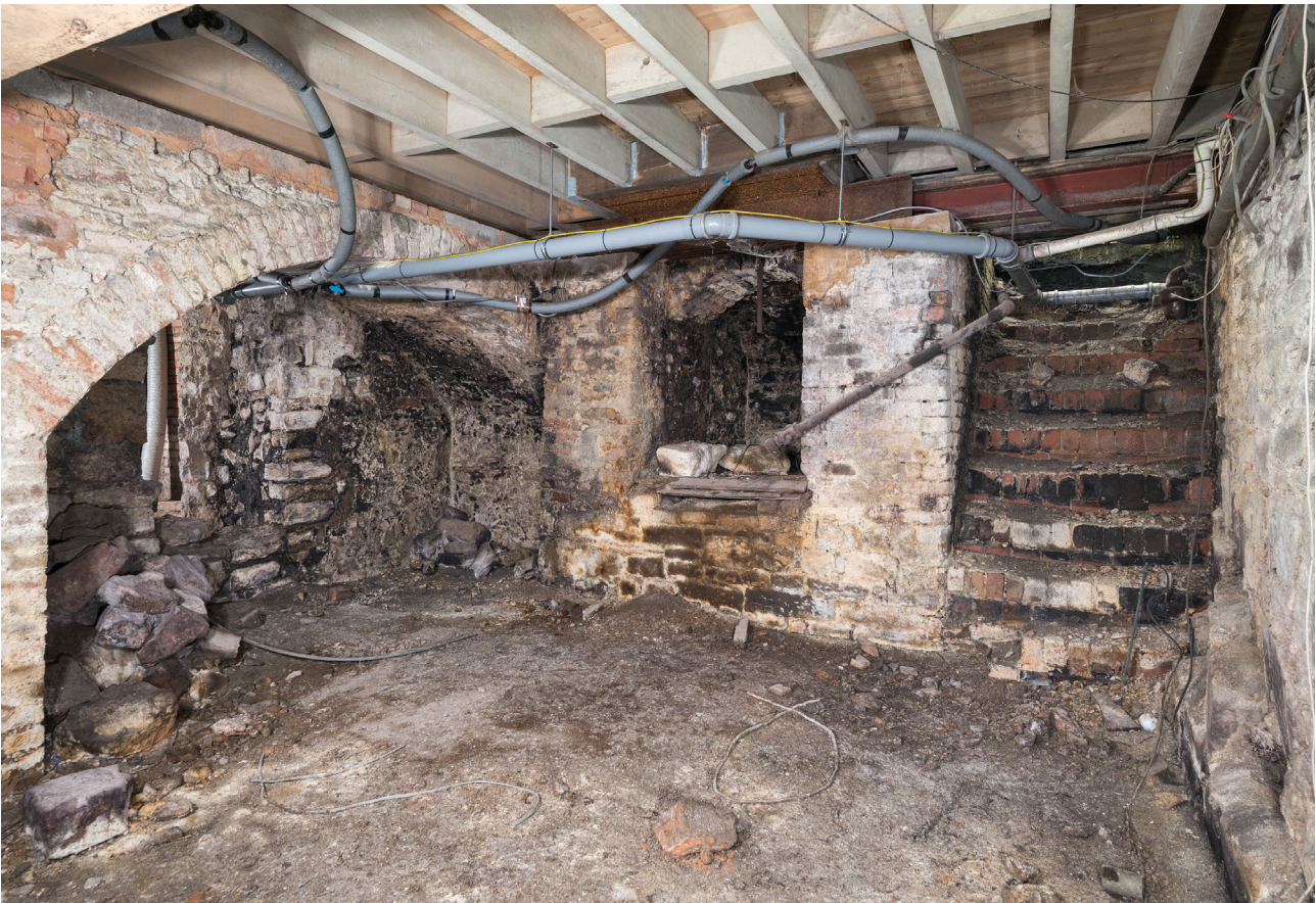
Figure 82: Looking at the south-eastern corner of the undercroft beneath no. 76 Westgate Street, showing brick stairs ascending in the south-western corner to street level. [DP325710]
