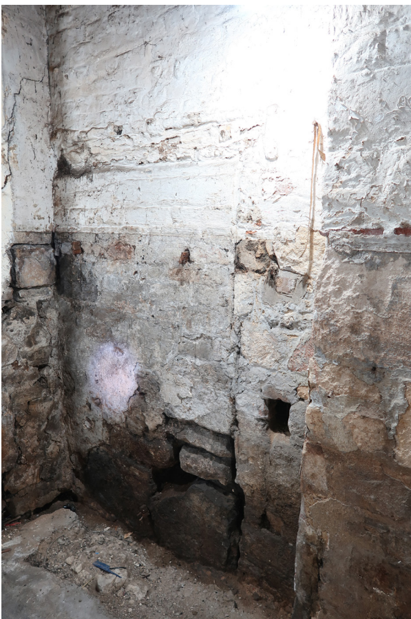
Figure 24: Blocked doorway with wooden lintel in the north-western corner of the undercroft at the Fleece. [Abigail Lloyd © Historic England]
