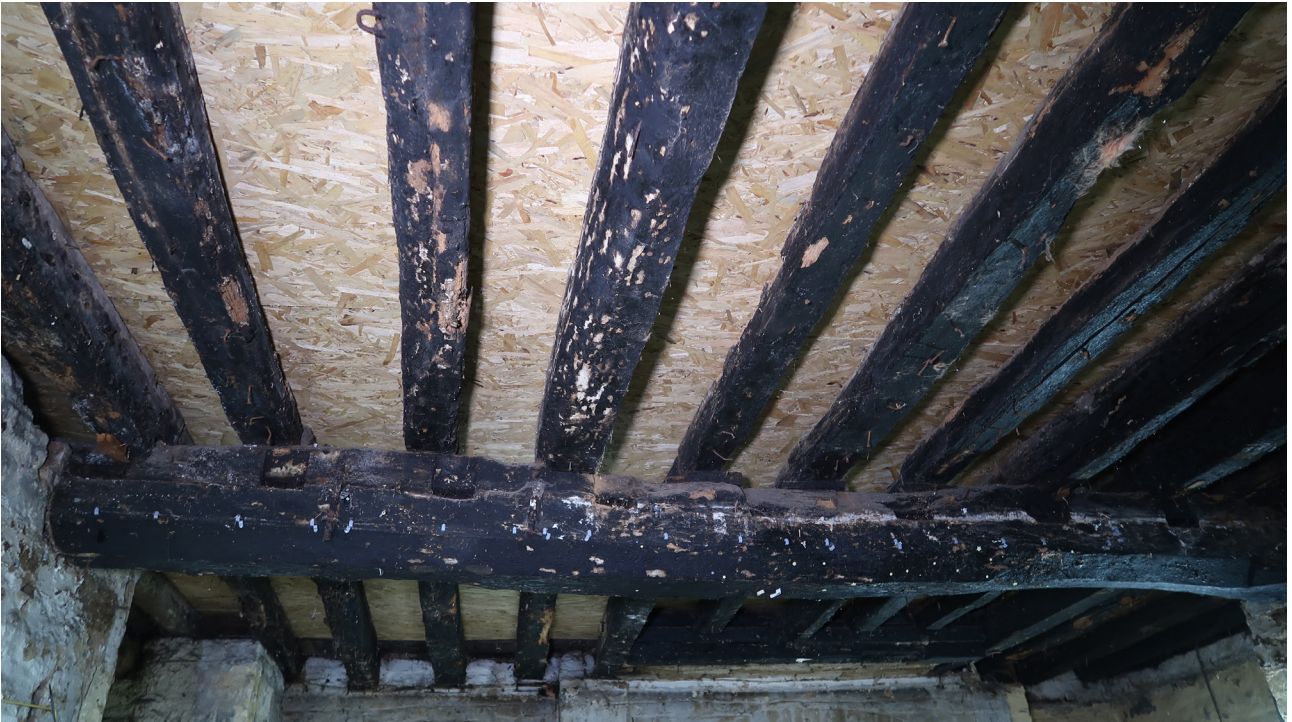
Figure 23: The transverse beam in the northern part of the undercroft at the Fleece, showing later joists laid on top of the beam and the mortices for earlier joists. [Abigail Lloyd © Historic England]
