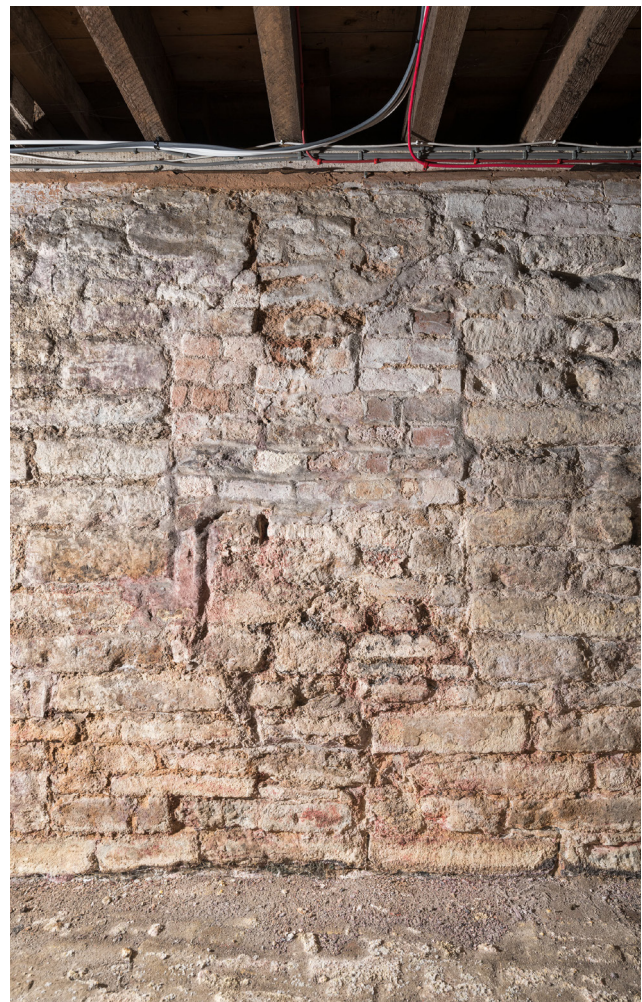
Figure 78: One of the blocked recesses on the eastern wall of the cellar under no. 74 Westgate Street. [DP325704]
