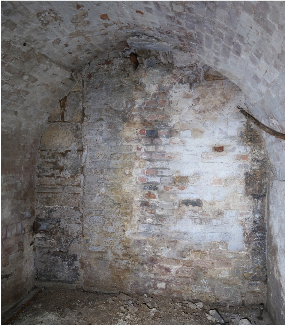
Figure 49: A blocked opening in the north-eastern corner of the street-front range at nos 47–49 Westgate Street, showing dressed quoin stones either side of brick infill. [Abigail Lloyd © Historic England]
