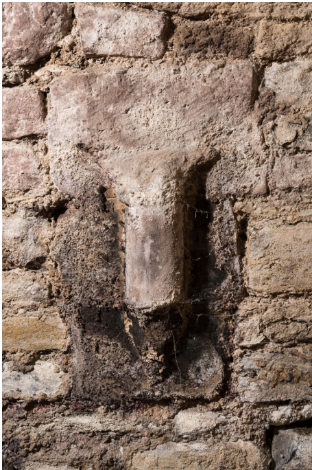
Figure 64: The eroded and partially removed fourth corbel from the north in the undercroft at no. 76 Westgate Street. [DP325711]
