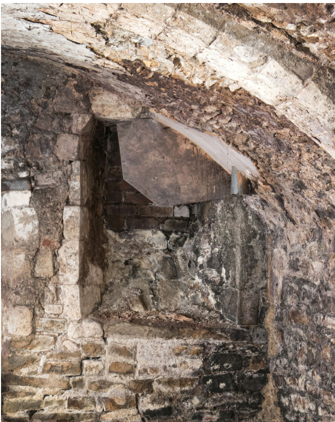
Figure 71: The north-eastern window in the undercroft at no. 76 Westgate Street, set at a higher level than the central opening. [DP325714 crop]
