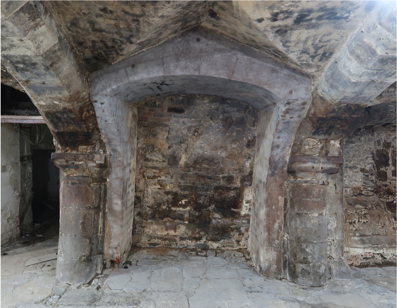
Figure 15: The wider bay 4 on the west side of the undercroft at the Fleece which was the primary entrance, now blocked and reinforced with later rendered brick framing. [Abigail Lloyd © Historic England]
