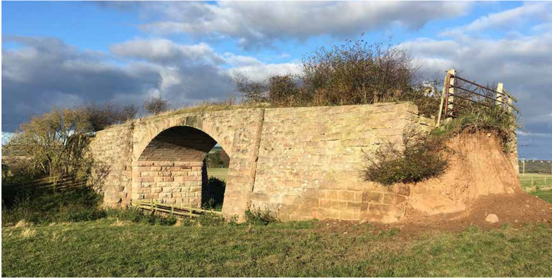
Figure 10: West-facing elevation of the truncated, masonry arch, accommodation bridge south of Chester Crane Camp, which used to provide access to the fields containing and surrounding the earthworks by carrying farm vehicles over the, now disused, Kelso to Tweedmouth branch railway line. [© Historic England]
