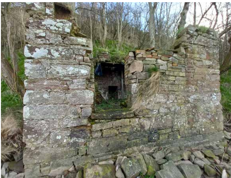
Figure 23: The north front wall and interior of the ruined Canny Shiel. March 2022. [© Historic England]
