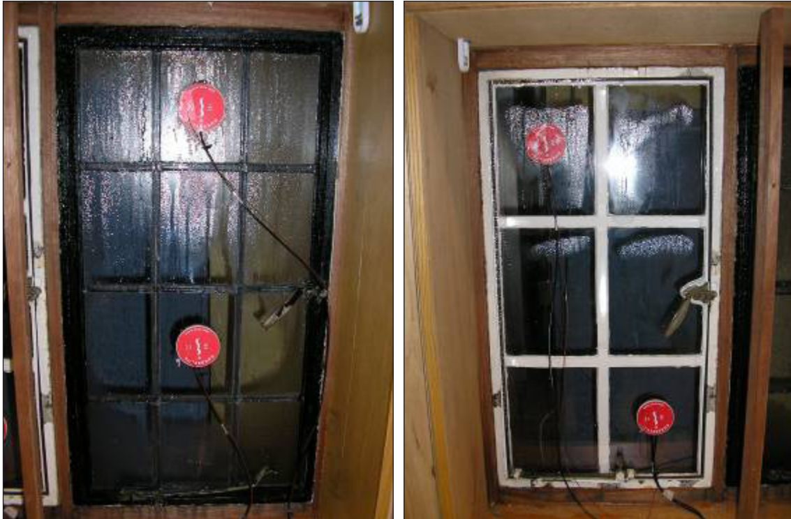
Figure 19 (left): Condensation on the black window.
