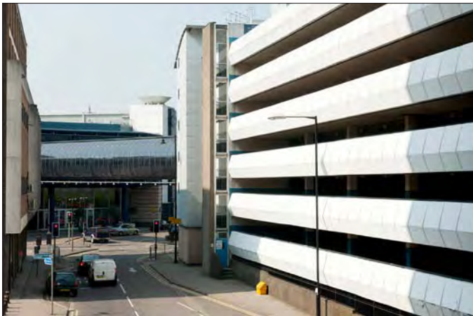
Figure 75. View of the rear of the Library Theatre car park. © Katie Carmichael.
