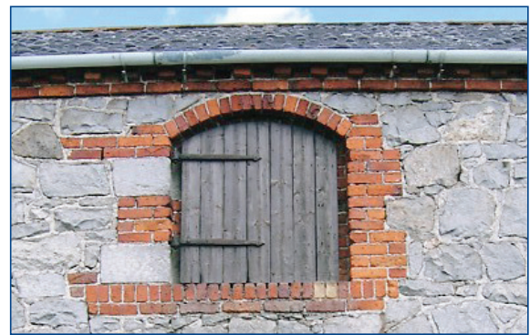
Stone rubble walling often has brick quins and dressing to window and door openings (Shropshire, Cheshire and Staffordshire Plain).
