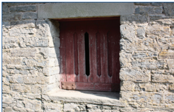
Hit and miss ventilation shutter – a characteristic feature of 19th century farm buildings (Shropshire, Cheshire and Staffordshire Plain).
