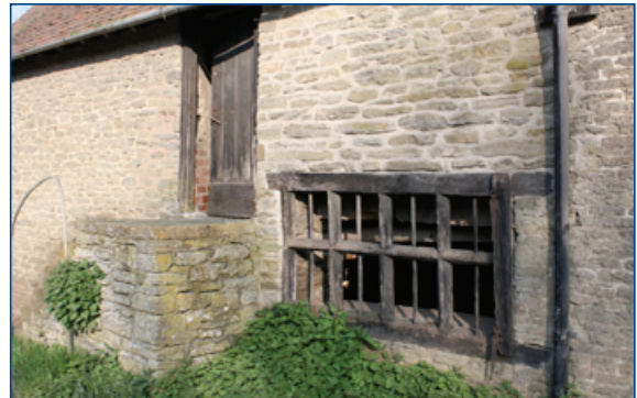
Timber mullion and transom window of late 17th or early 18th century date (Shropshire Hills).
