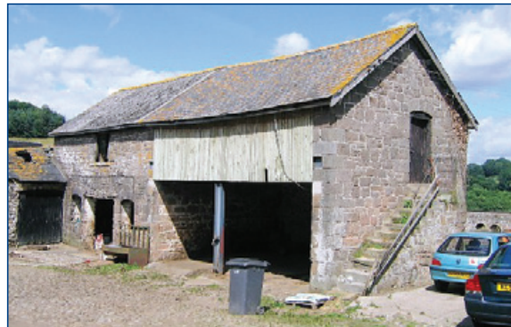
Cartshed with granary over allowing carts to be loaded directly from the granary. This cartshed adjoins a stable and faces onto a road running alongside the farmstead (Oswestry Hills).
