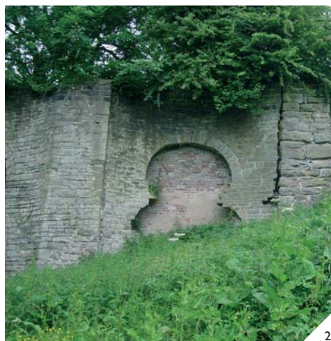
2 Stockport, Greater Manchester: a neglected bank of lime kilns, one of which is being forced apart by scrub growth. The land, set apart for display of the monument, has no information panels.
