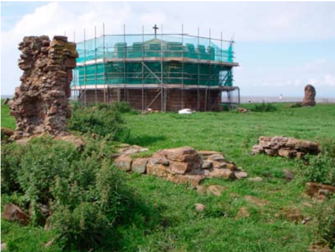
View of standing remains around the chapter house showing conservation work in progress
