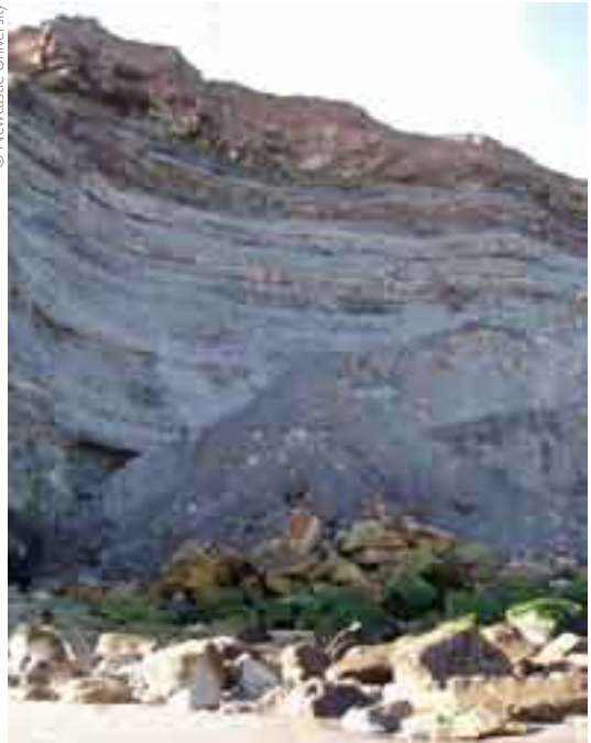
Failed cliff material corresponding to Feature C
