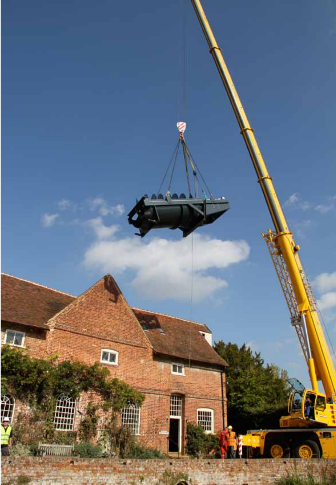
Lifting the turbine over the building at Flatford Mill (Photo courtesy of MannPower)
