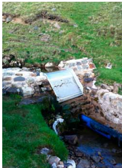
Penstock (blue pipe) leaving a coanda screen (Photo courtesy of Dulas Ltd)
