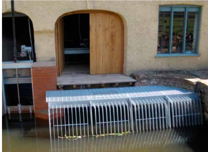
Forebay tank and trashrack (photo courtesy of Stephen Bartlett)
