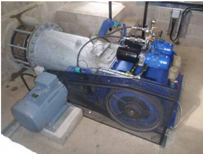
Generator connection (Photo courtesy of MannPower)
