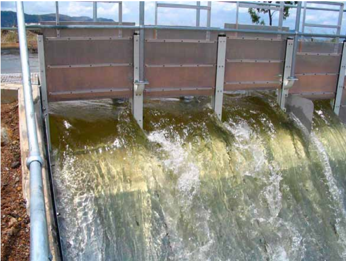
Sluice gates over a coanda screen (Bilfinger Water Technologies Ltd)
