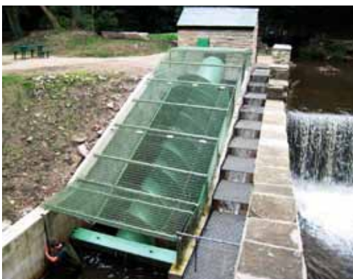
Archimedes Screw turbine and fishrun at New Mills (Photo courtesy of MannPower Consulting Ltd)
