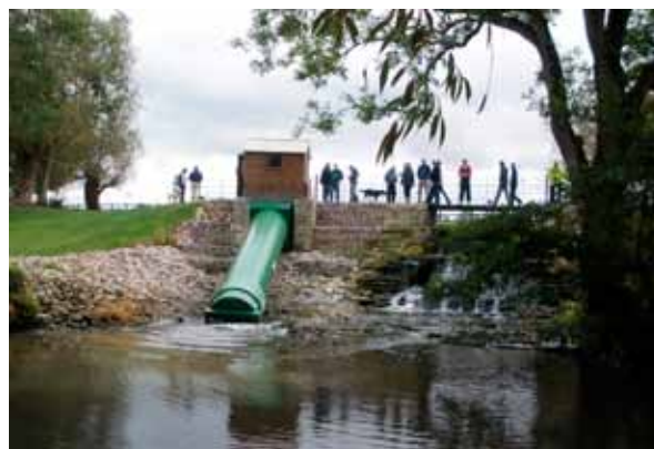
Archimedes screw turbine (Photo courtesy of Stephen Bartlett)
