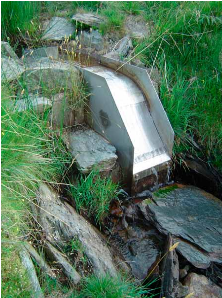
Coanda screen (Photo courtesy of Dulas Ltd)
