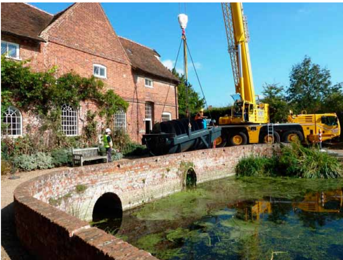
The arrival of the turbine at Flatford Mill (Photo courtesy of MannPower)
