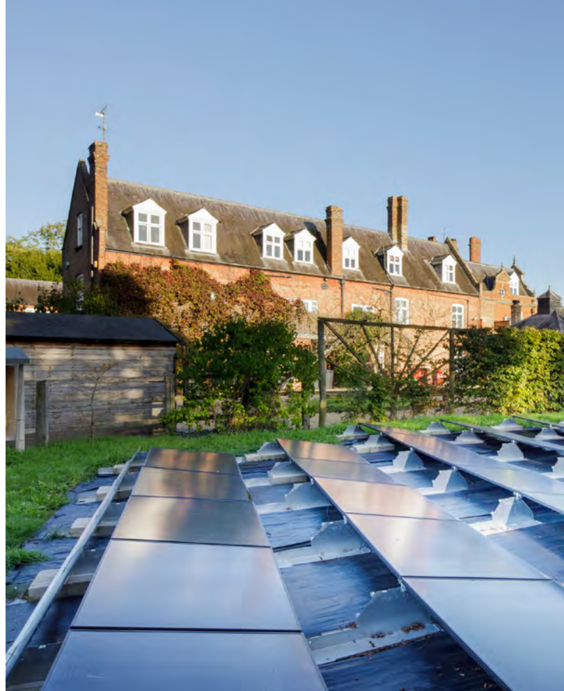
Chippenham Hall, Chippenham, Cambridgeshire. Solar panels have been installed in the garden.
