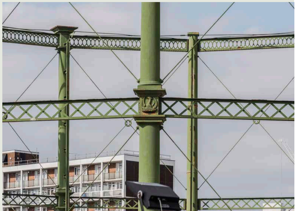
Figure 10: Photography should also be used to capture architectural and structural details, such as this phoenix emblem on number 2 gasholder at the Phoenix Gas Light and Coke Company's Kennington Lane works. [DP182538]
