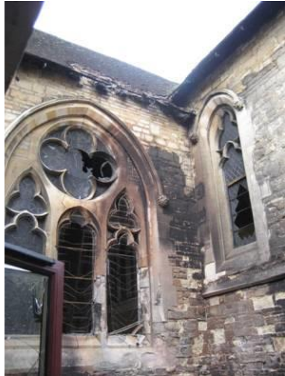
Damage caused by shed on fire
