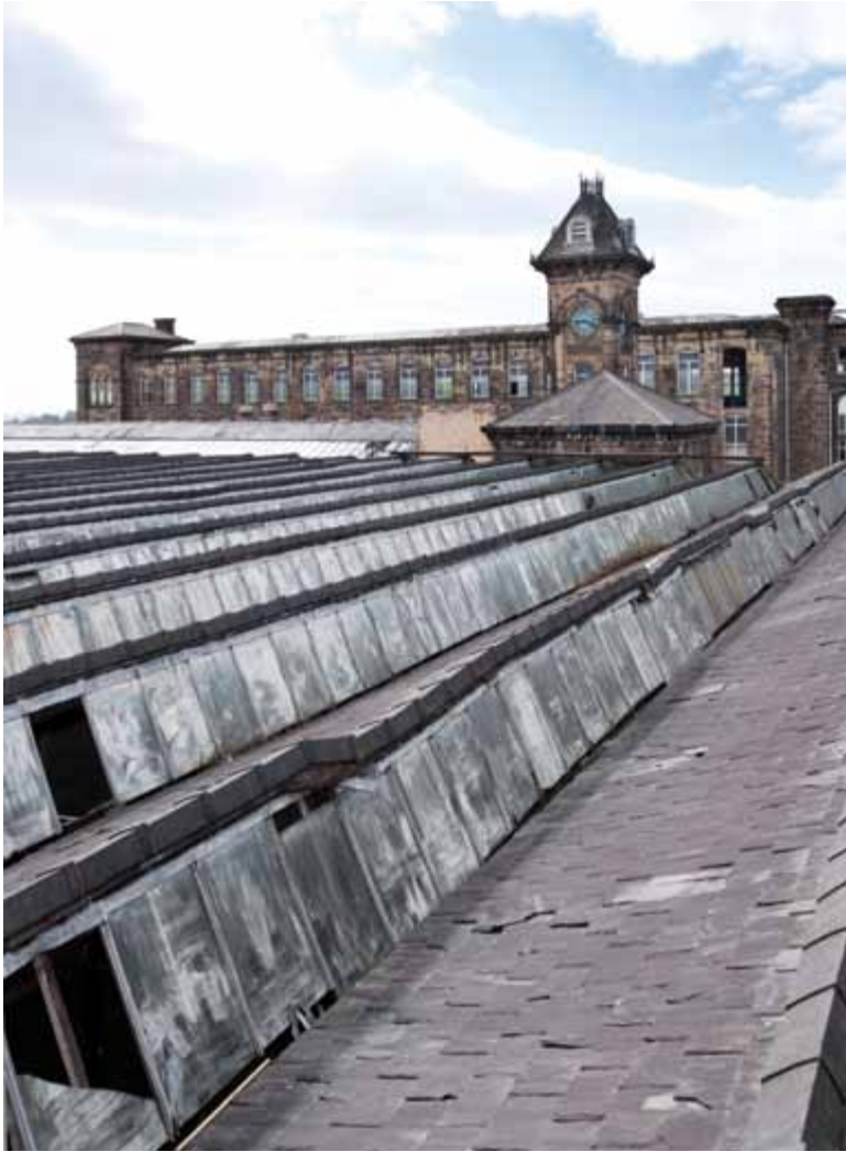
Top left: North-light roofs in need of repair
