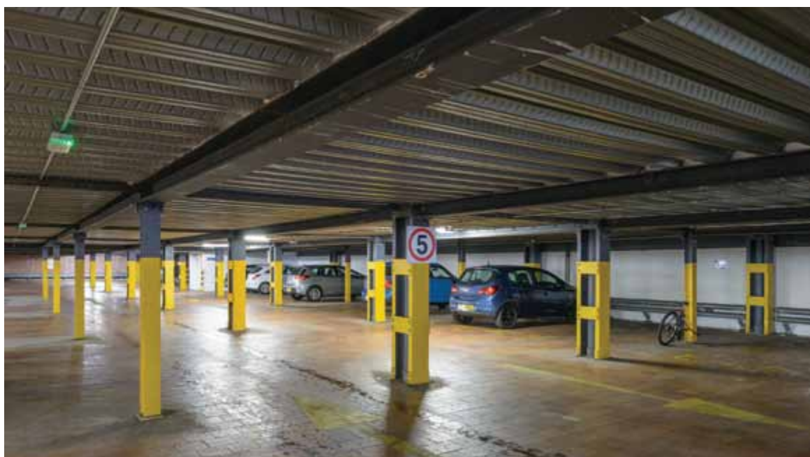
Undercroft car parking was created in addition to surface car parking due to the number of residential units being created
