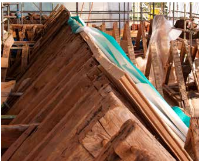
Figure 2 (above): Insulation above the rafters only Insulation here is shown only on top of the rafters if it was not considered possible to place insulation between the rafters as well. An air path is provided above the sarking insulation by counter-battening. The use of thicker sarking insulation together with counter-battening could raise the roof by at least 75mm which might pose a number of detailing problems.
