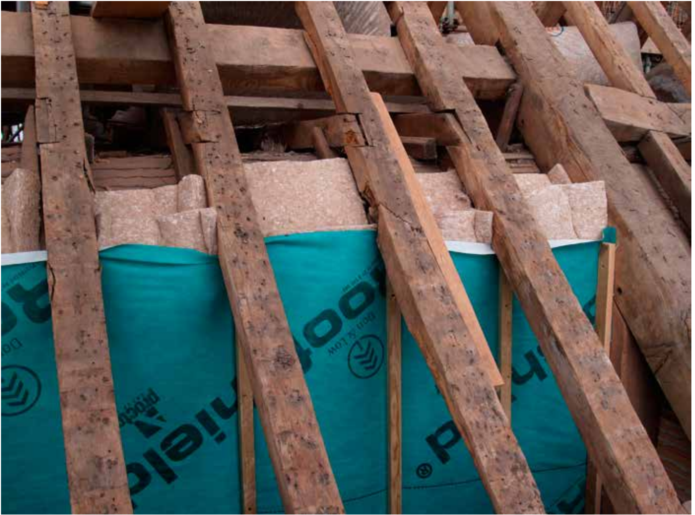
Figure 16 Sheep's wool insulation with a vapour permeable membrane added close to the eaves. © Oxley Conservation
