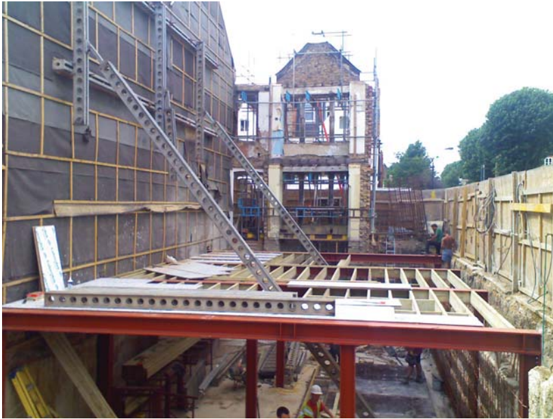
This unlisted building in a London conservation area was effectively demolished without consent, apart from the front façade, resulting in a record fine of £120,000 and costs of £100,000 awarded to the Council. The works to excavate a new basement commenced before planning approval had been given and instability to the flank and rear walls ensued. © Bob Kindred
