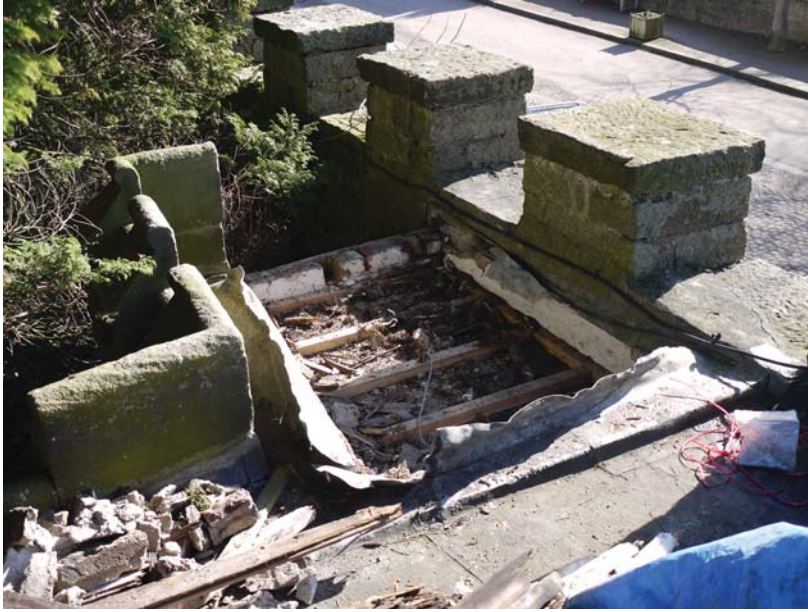
The gatehouse roof at Ripley Castle in North Yorkshire, following the theft of lead in 2011. The occupants were on holiday when the lead was taken and the subsequent water ingress caused considerable internal damage.
