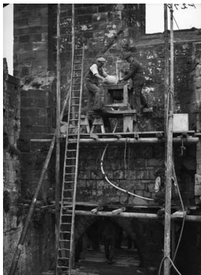
Repairing the walls of Furness Abbey, Cumbria, in the 1920s, using a gravity grouting machine.
