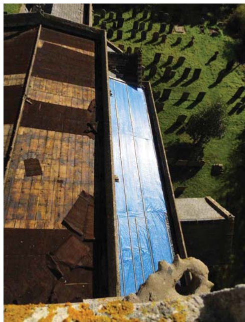
The roof of the Grade II* Church of St Bartholomew at Sproxton in Leicestershire after an attack by metal thieves.
