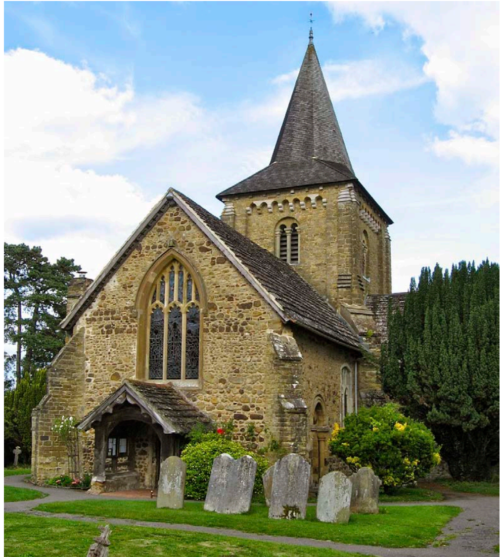
Figure 23: Church of SS Peter and Paul, Ewhurst. Wealden Sandstone blocks and rubblestone with occasional blocks of ironstone (carstone); Horsham Stone slate roof.
