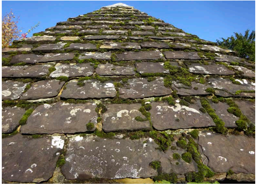
Figure 72: Lych gate roof, Church of St James, Shere. Horsham Stone slate roof.
