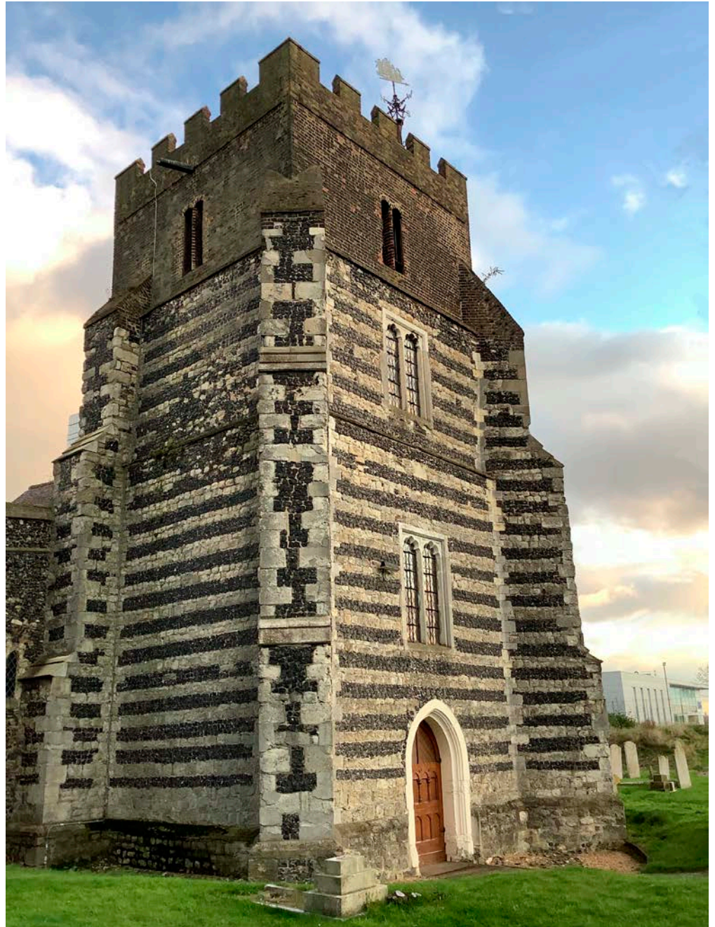
Figure 12: Church of St Clements, West Thurrock. Quarry Flint and Kentish Ragstone banding with Reigate Stone dressings.
