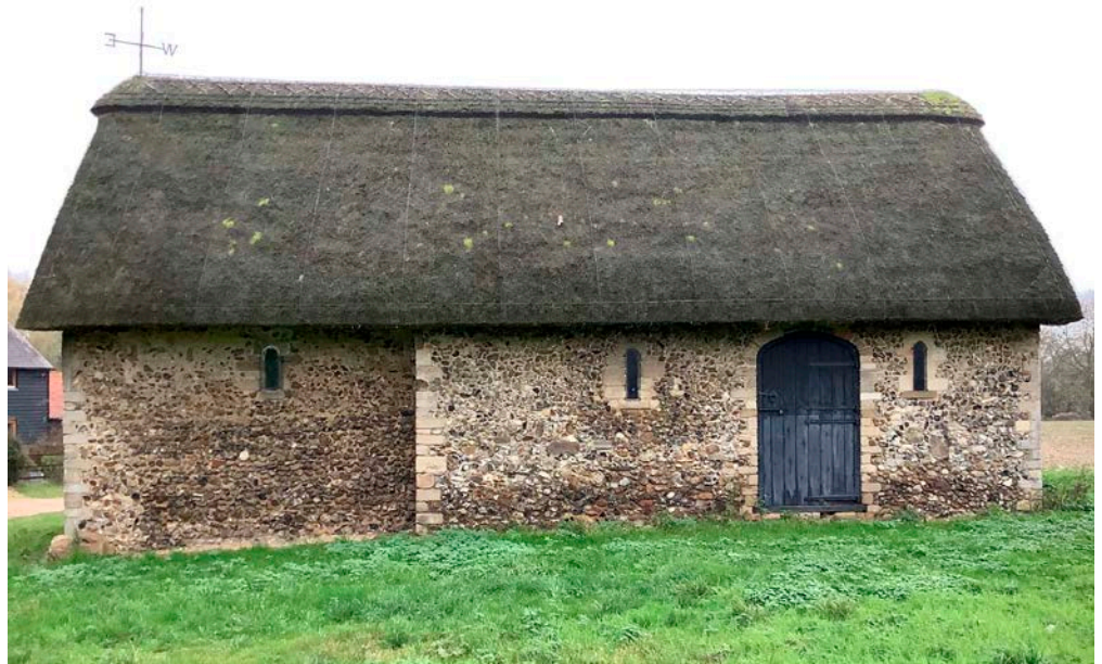
Figure 39: Former Chapel of St Helen, Wicken Bonhunt. Sarsen stone with Hertfordshire Puddingstone, pebbles and cobbles.
