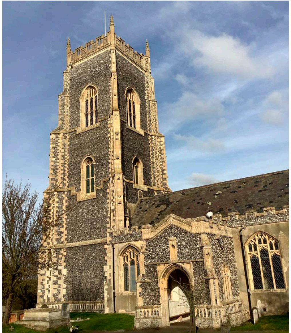
Figure 47: Church of All Saints, Brightlingsea. Knapped Quaternary Flint with Bath Stone dressings, and possibly some Lincolnshire Limestone.
