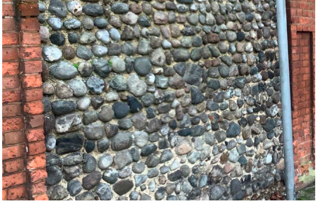
Figure 70: Roadside wall, High Street, Mistley. Igneous and metamorphic rocks, some from the Larvik area of Norway.
