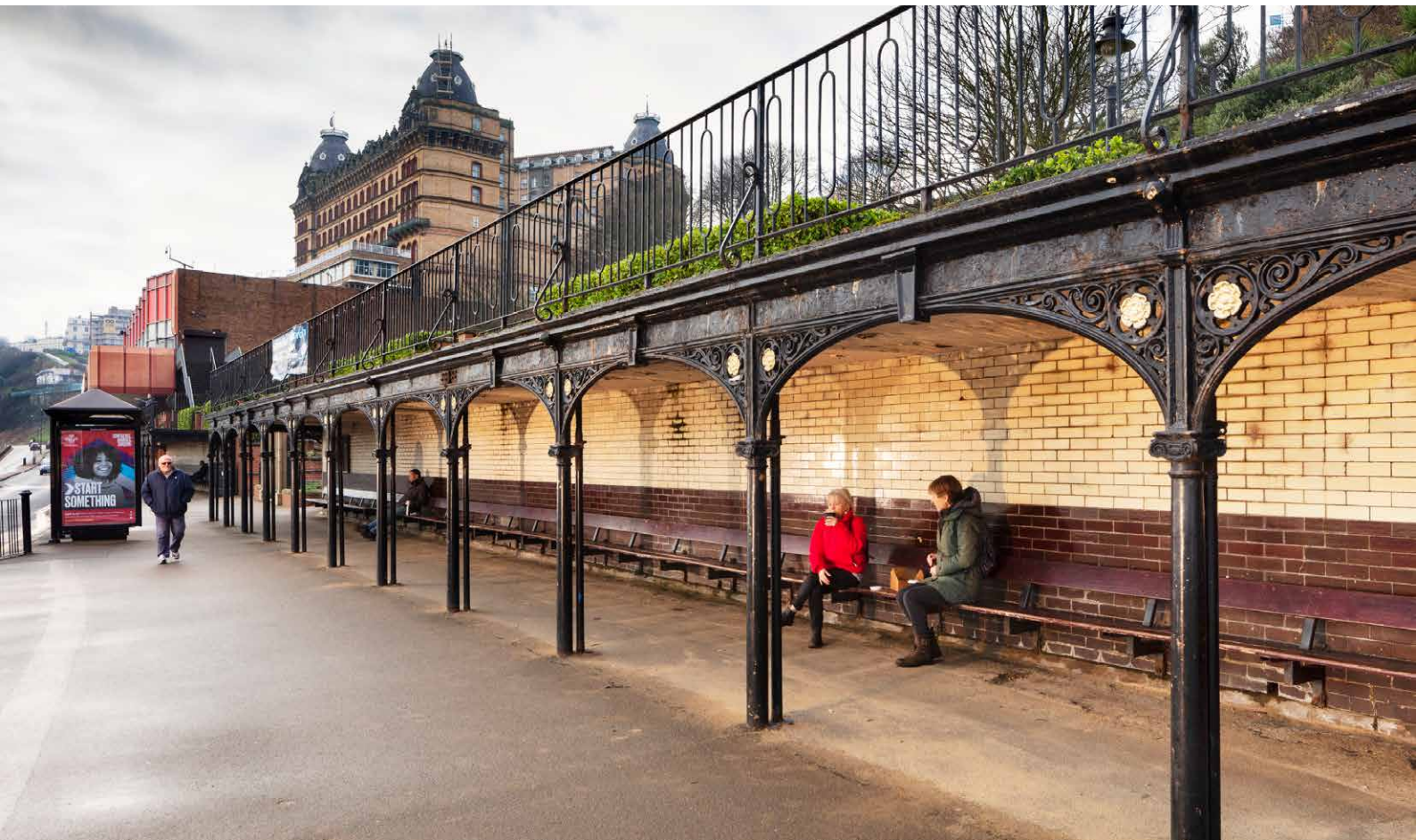
Seating shelter and viewing terrace to front of St Nicholas Gardens, Scarborough, North Yorkshire. © Historic England Archive
