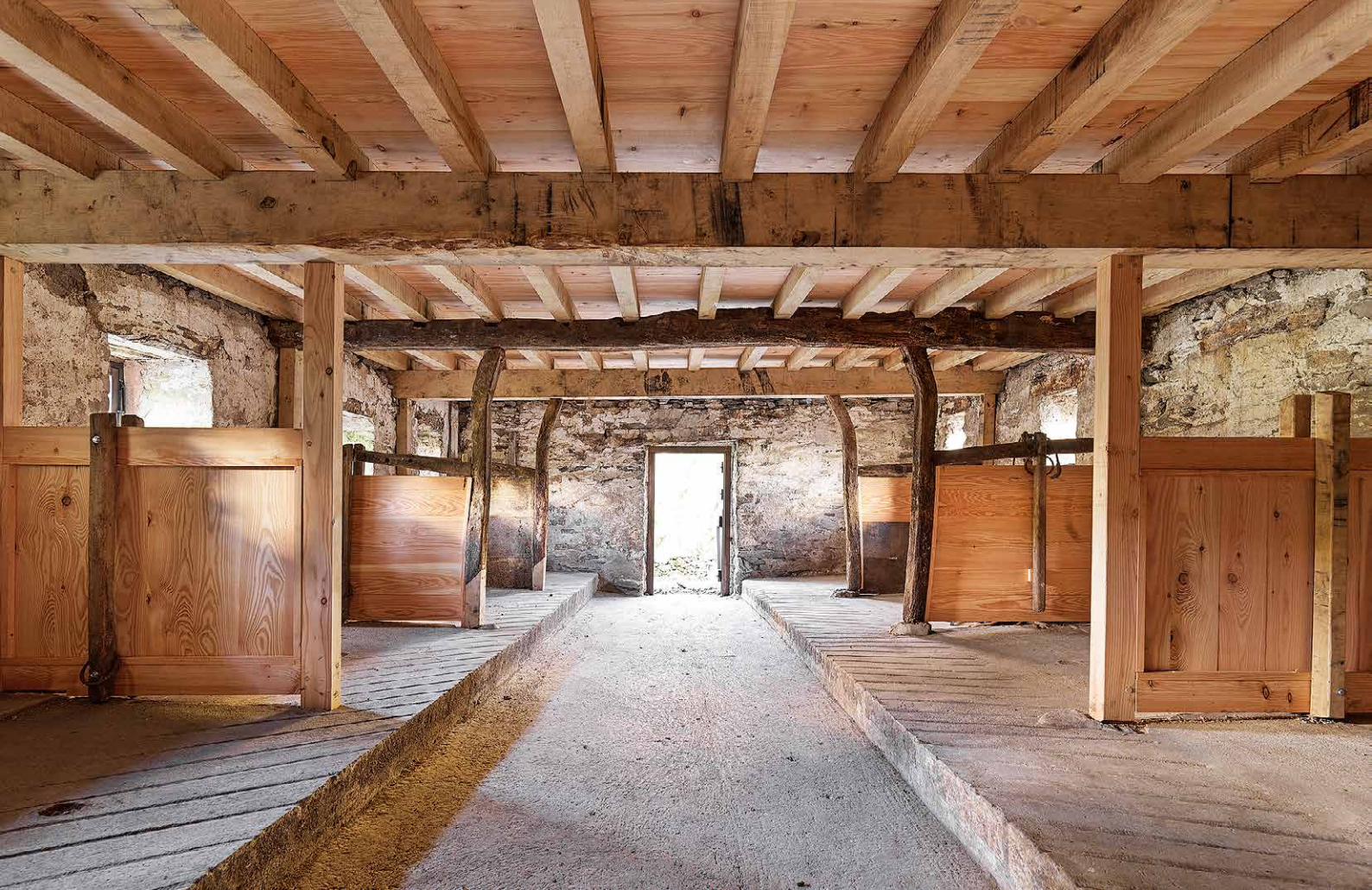
National Parks Pilot Scheme for Field Barns: Newly installed field barn, Bridge End Farm, Longsleddale, Cumbria. © Historic England Archive
