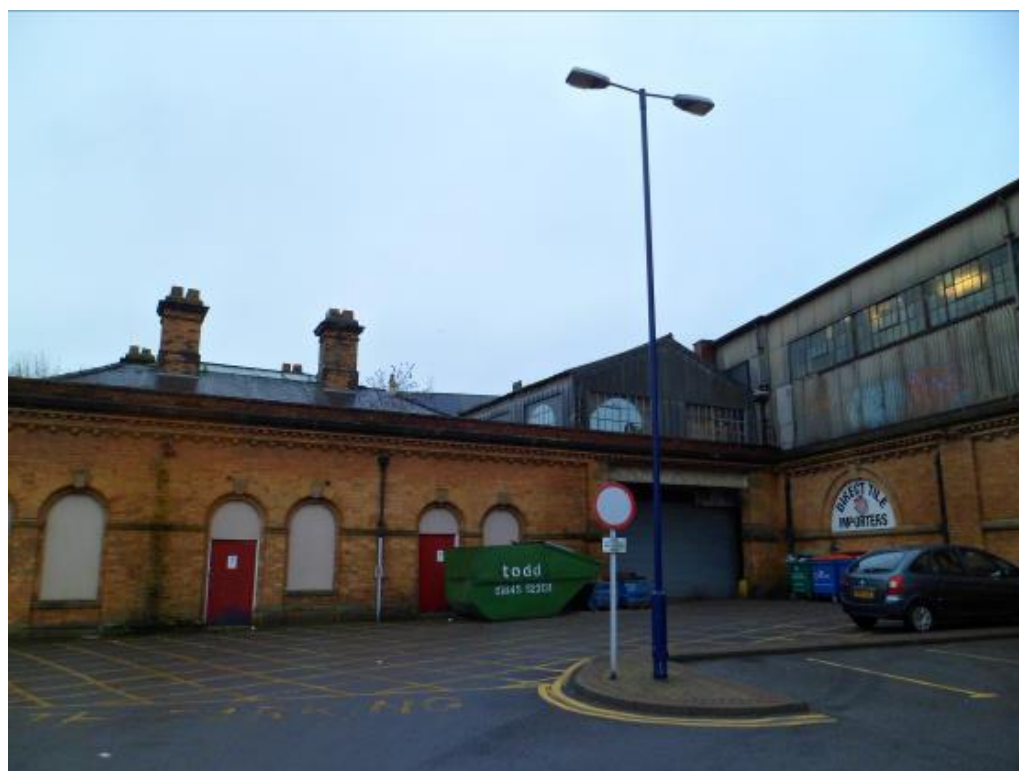
The building before repair (Photo: © Scarborough Studios Ltd).
